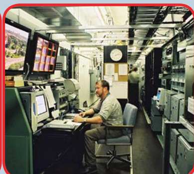
Central office, 1990's
